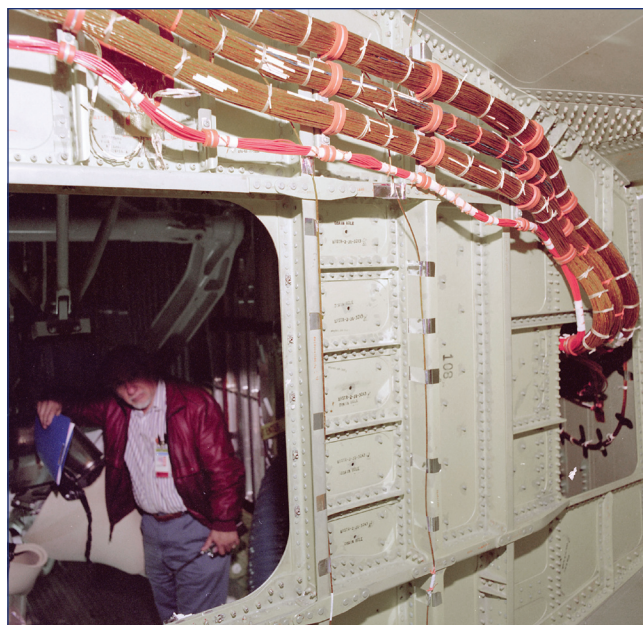
Figure 4.2-3. Typical wiring bundle inside Orbiter wing.
